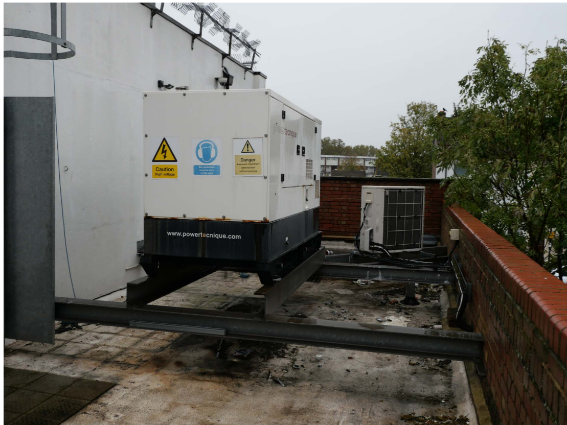
1st fl. roof terrace to east with AC plant
